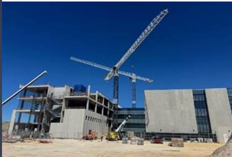
SSN Training Centre looking West. Full eastern elevation showing precast panel installation commencement to perimeter.
